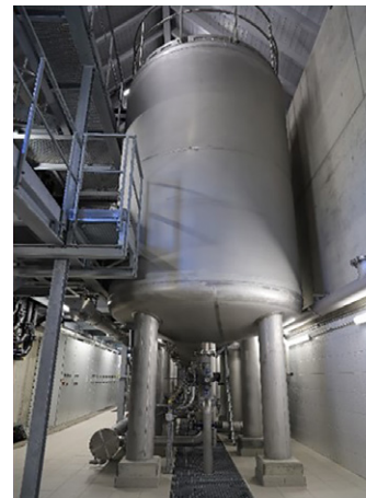
Activated carbon filtration system used for PFAS contaminated water treatment
