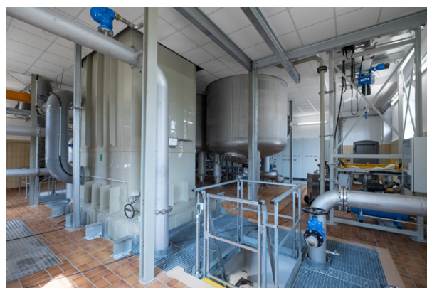
The current treatment solution at the Rauental waterworks
