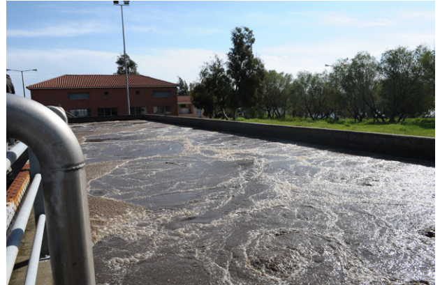
Activated sludge bioreactor for municipal wastewater treatment at the Mytilene STP
